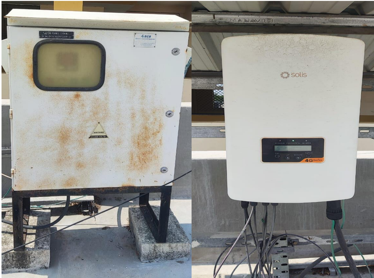
Figure 7 Solar PV Roof Top System
