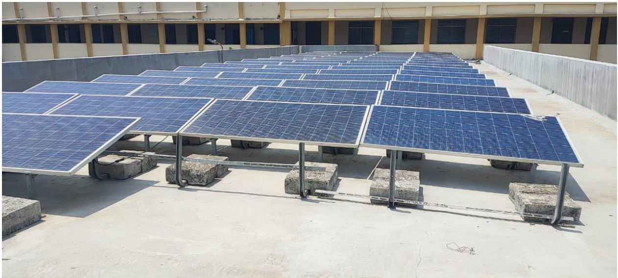
Figure 6 Solar PV Roof Top System
